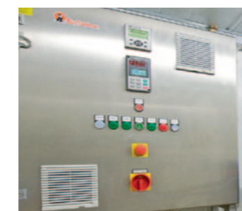
Individually planned control box
